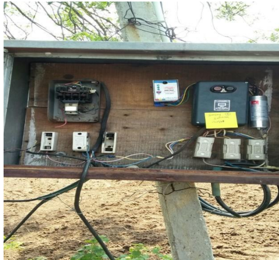
Fig. 4 Capacitor connected at the pump terminal
