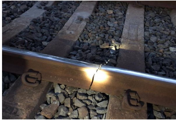
Fig. 3 Image of Track with crack
